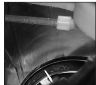
Properly adjusted TXV
