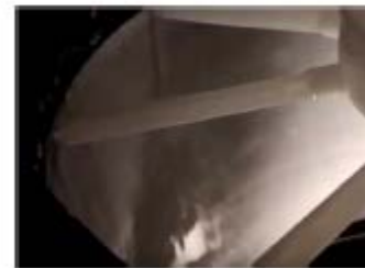
Properly adjusted TXV
